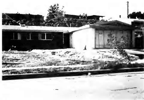
Photo 17. View west across Newton Street showing scarp about 30 cm (12 inches) high along fault break of Sylmar segment of San Fernando fault zone. Break extends into southwest edge of house which was later razed. Most houses along fault break in this neighborhood have been razed; most houses on southern side of fault were not badly damaged, but houses on north (up-faulted) side were generally badly damaged, though repairable. Houses partly or wholly on fills in this area commonly were damaged by the effects of shaking.
